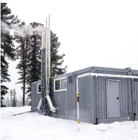
INSTALLATION IN KALTEN KLIMAZONEN
